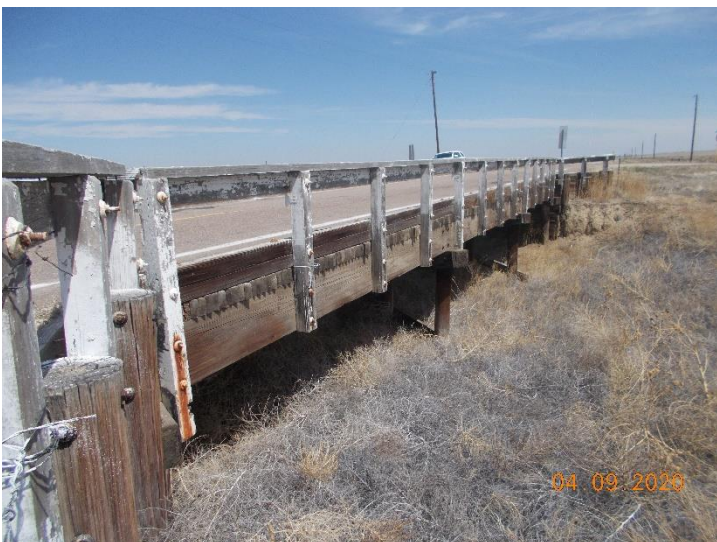
View of bridge M-21-I looking northeast along the south side of the structure showing the extent of the lead-based paint.
